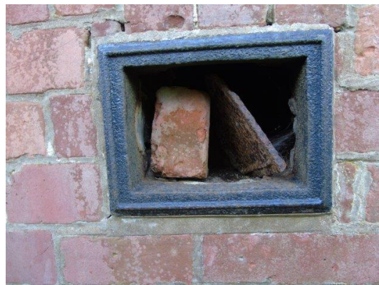
Open vent with missing insect pest grill
