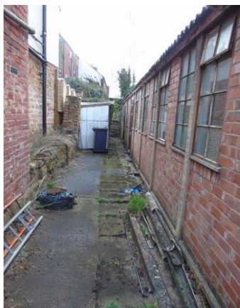
Asbestos pipe waste
