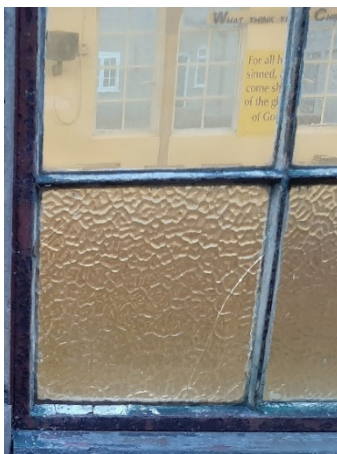
Poor putty and cracked pane
