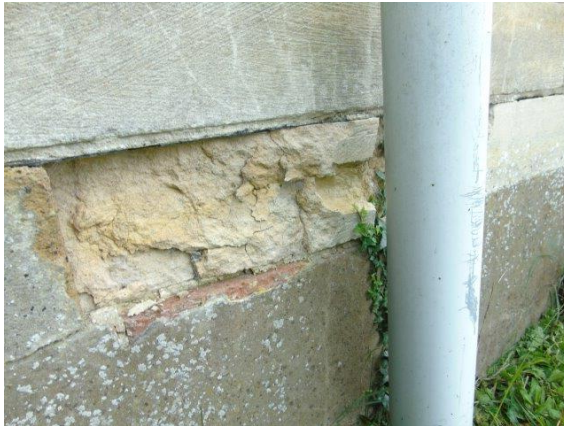
Spalling of stonework
