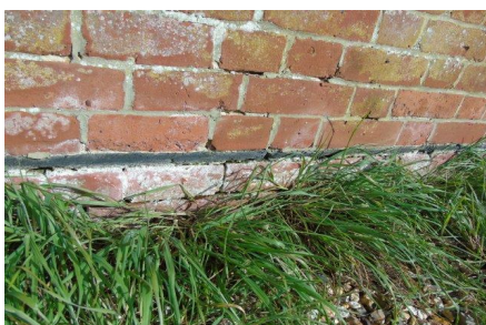
Historic DPC material in poor condition
