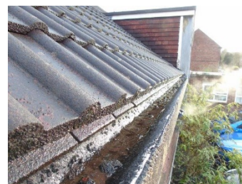
Debris in concrete gutter
