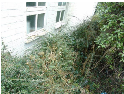
Overgrown area next to building
