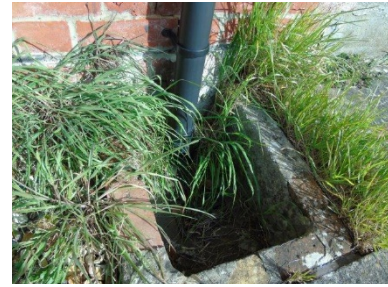
Blocked overgrown gully
