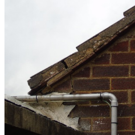
Verge - poor pointing
