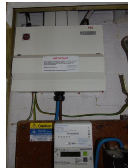
Electrics - inspection date sticker
