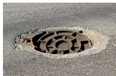
Broken manhole cover
