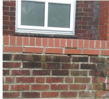
Mortar missing to brickwork
