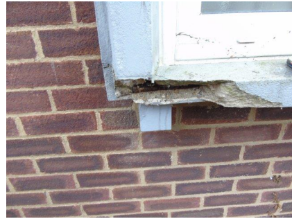
Concrete frame cracked open
