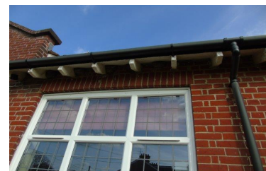
Exposed rafter needing painting
