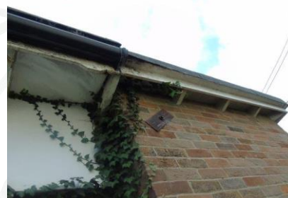
Ivy ingress and damage to external wall and soffit
