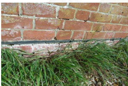
Historic DPC material in poor condition
