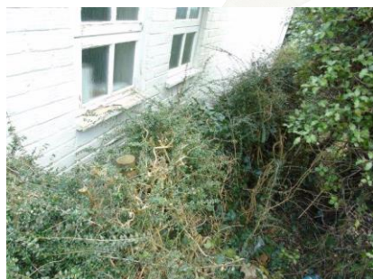
Overgrown area next to building
