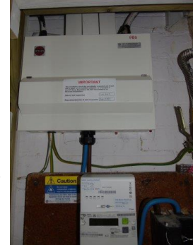
Electrics - inspection date sticker
