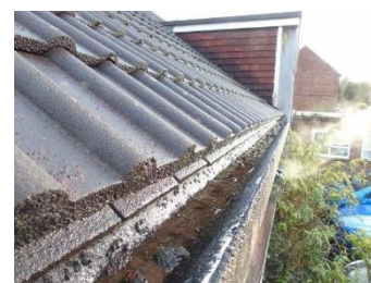
Debris in concrete gutter
