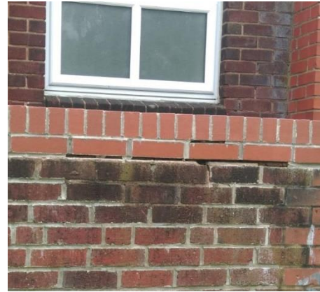
Mortar missing to brickwork
