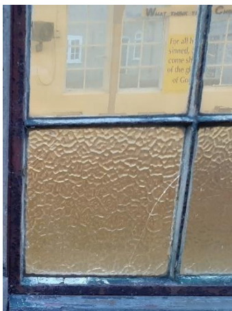
Poor putty and cracked pane
