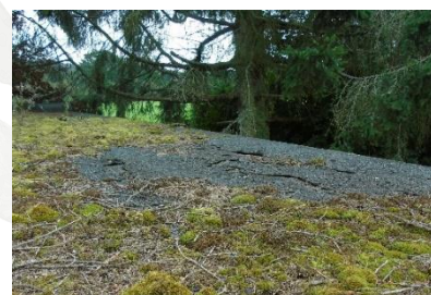
Moss and tree debris gathering on flat roof and cracking of roof
