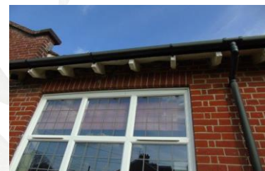
Exposed rafter needing painting
