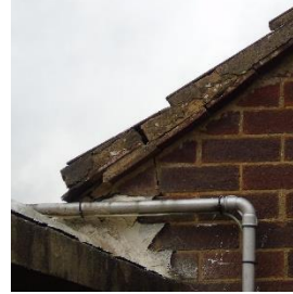
Verge - poor pointing
