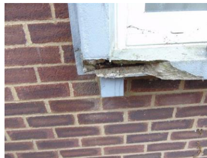
Concrete frame cracked open
