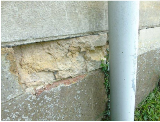
Spalling of stonework
