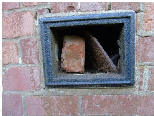
Open vent with missing insect pest grill
