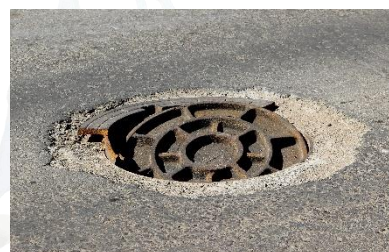
Broken manhole cover
