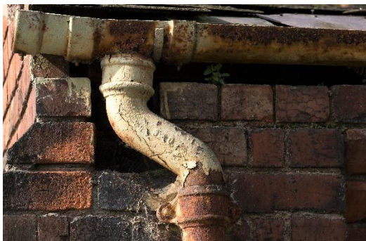
Cast iron gutter
