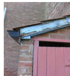
Timber bargeboard in poor condition
