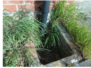
Blocked overgrown gully
