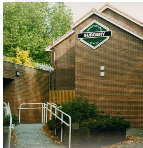
Figure 6: Example of a lower handrail being installed to facilitate use by children or persons of a low stature.
